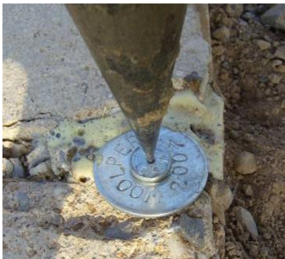
Figure 5-40. Provides a close up of the nail and washer marking the Runway Direction feature location.
