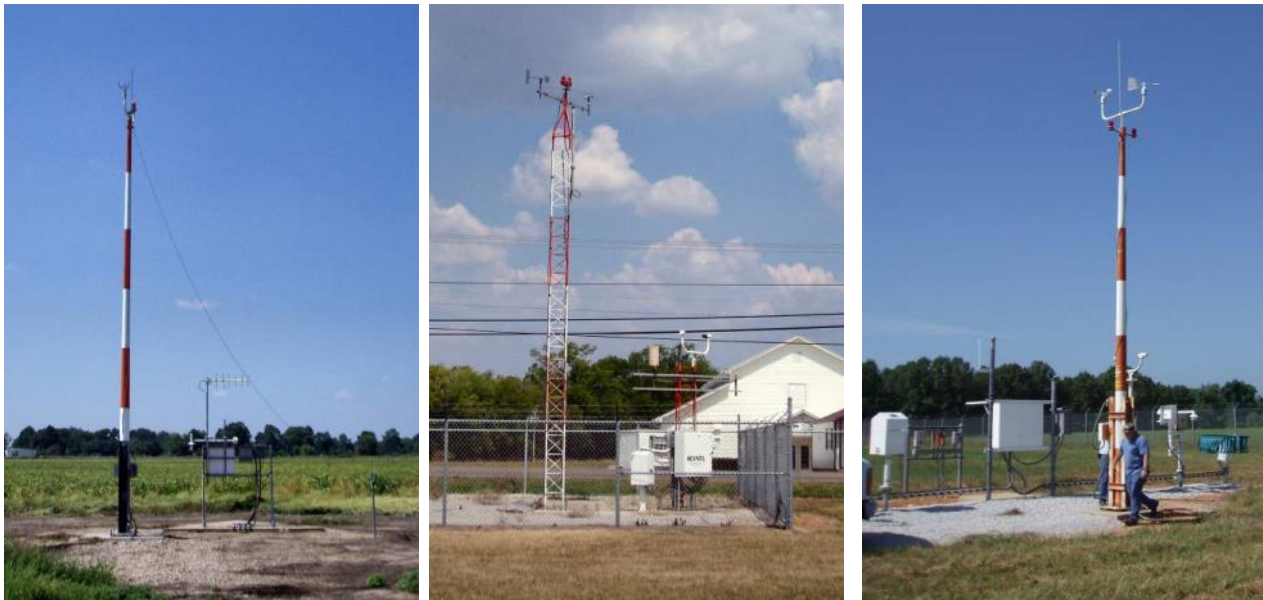
Figure 2-16. SAWS, AWOS and ASOS Station Installations
