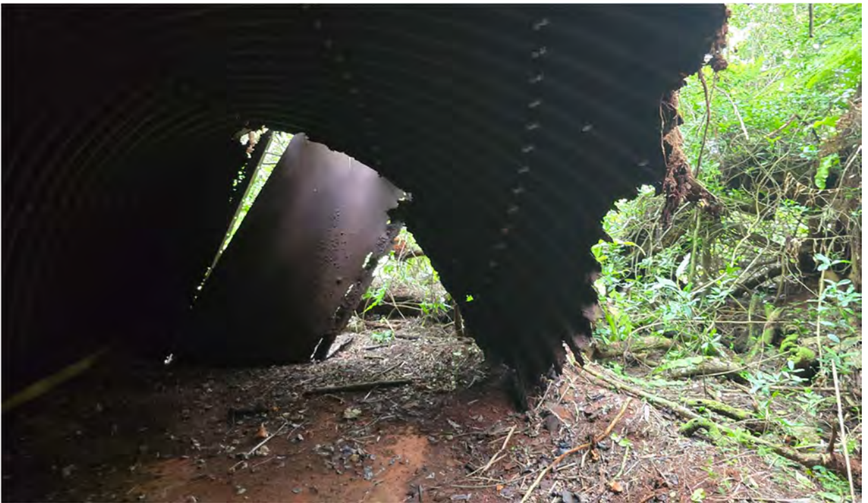
Figure 18: View from interior of TS-1 showing partially collapsed Quonset.
