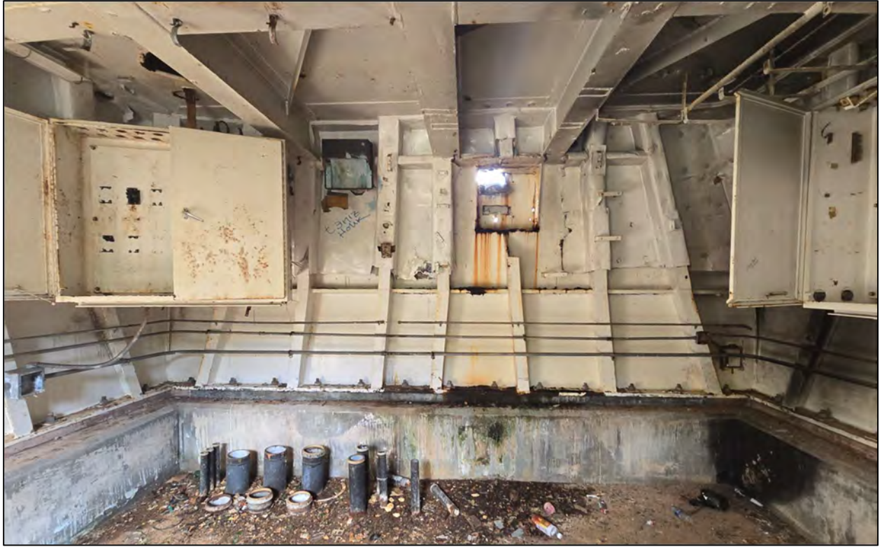
Figure 29: View of interior of radar - accessed through door.
