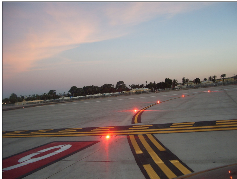
FIGAD 1.1-10 Runway Entrance Lights
