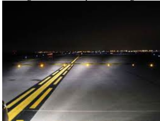
Figure 2: Runway Guard Lights
