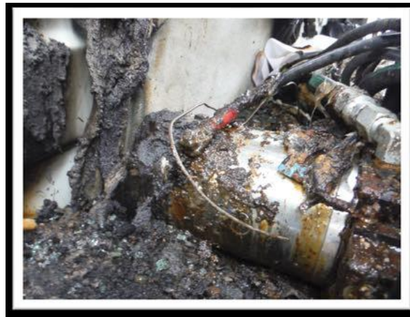
Aftermath of September 29, 2016, fire
