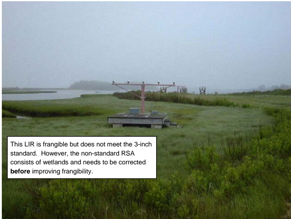
Non-Frangible NAVAID installed in an RSA that does not meet standards.
