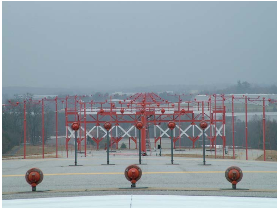
Standard ALS installation. Note electrical metallic tubing (EMT) with frangible couplings installed on light stations that are less than 6 feet high.
