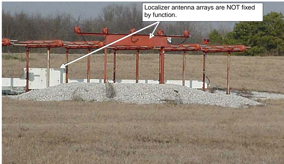
Excessive gravel fill creates a hazard
