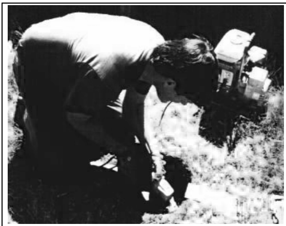
Figure 8.22. Cutting off the top of the stainless steel rod using a hydraulic cutter approximately 3 inches below the surface.
