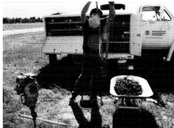
Figure 7-12. Digging the 43" deep hole; 12"-14" diameter for the top 22" in depth, and 3"-6" diameter for the bottom 21".
