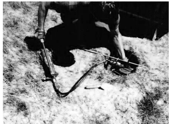
Figure 7-15. Cutting off the top of the stainless steel rod using a hydraulic cutter approximately 3 inches below the surface.
