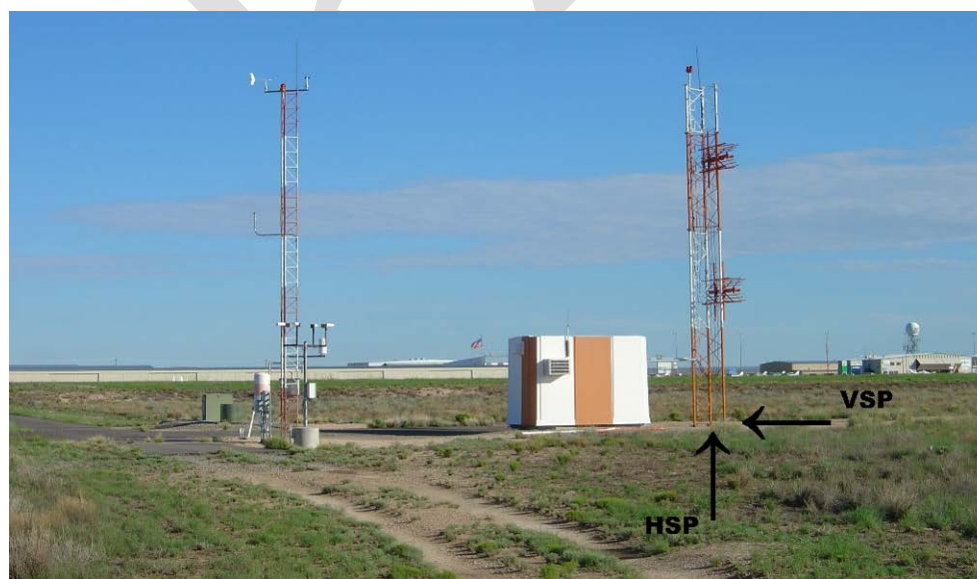
Figure C-6. Typical glideslope installation.
