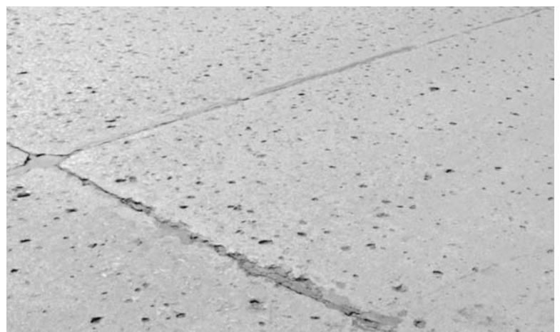
▶ Extensive pop-outs of large aggregate from surface.
