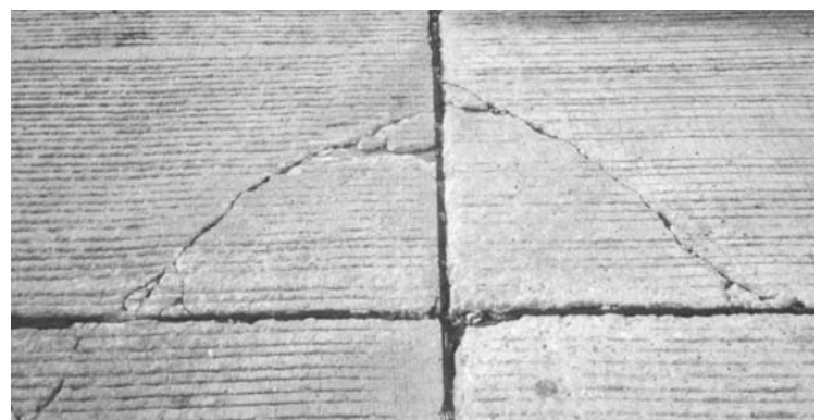
Corner cracking with slight spalling.
