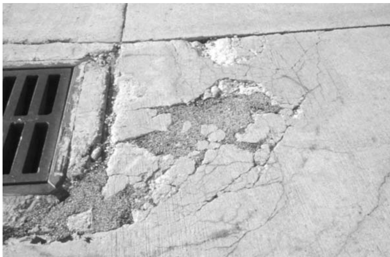
▼ Inlet with severe cracking and spalling. Full depth slab repair required.
