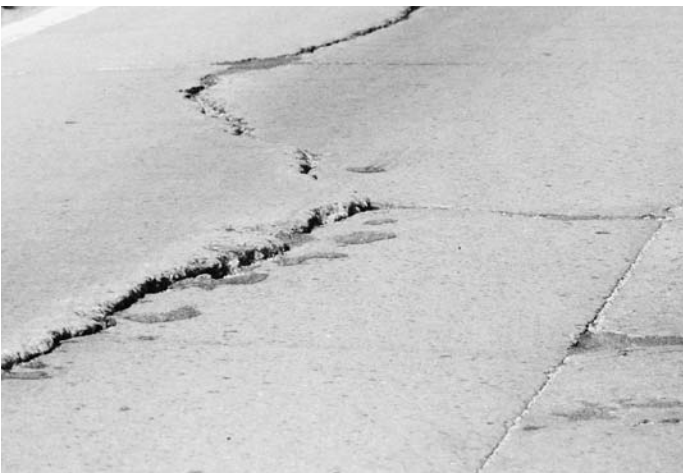
◀ Faulting and spalling of a meander crack.
