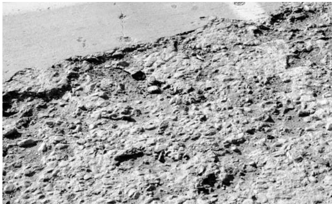
▶ Moderate surface scaling. Loss of mortar and fines starting to expose larger aggregate.
