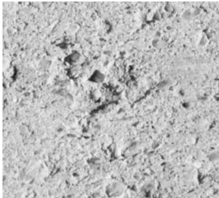
▲ Slight scaling. Minor loss of surface mortar.
