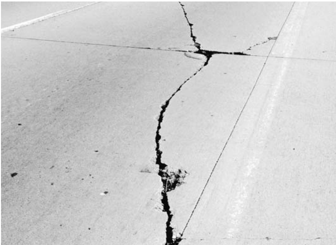
◀ Meander crack caused by settlement. Lack of maintenance allows water to intrude and debris to collect in crack.
