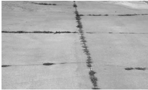
▲ Open joints and cracks. Need sealant on more than 10% of joints.
