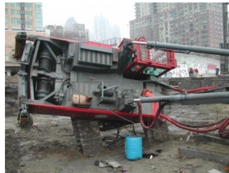
Figure 4: A crawler crane relies on firm level ground support to keep it from tipping.
