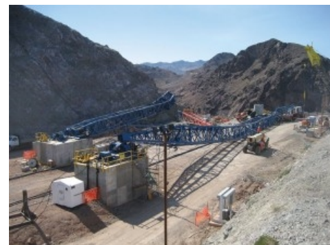
Figure 6: A half-mile-long cableway across Black Canyon on the Colorado River collapsed during high winds. Its loss set back construction of a vital interstate bridge link by two years.
