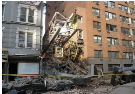
Figure 5: On the Upper East Side of Manhattan, a tower crane collapsed during a climbing operation, resulting in multiple deaths and massive property damage.
