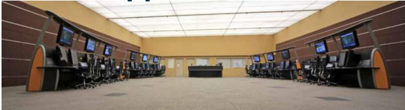
AREA Control Centre
