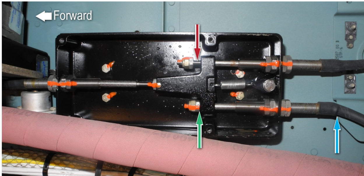
Figure 8. View inside the junction box for the accident helicopter's emergency flotation system.
